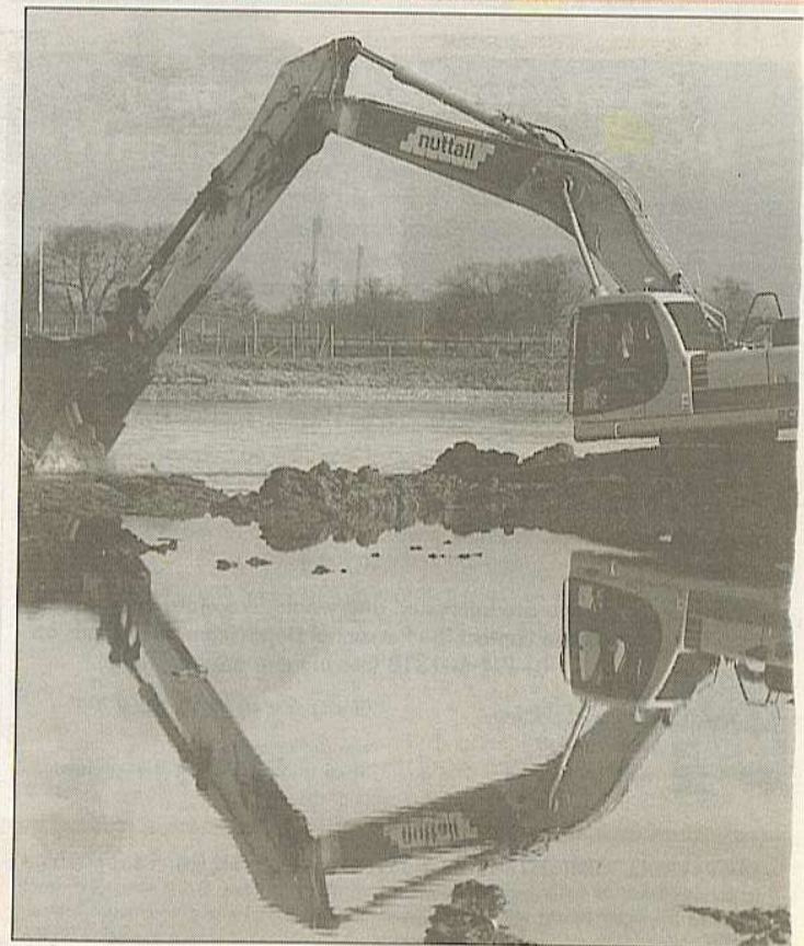
■ THE JUBILEE RIVER: The Maidenhead & Windsor Flood Alleviation Scheme, the area's biggest construction project in recent years.
